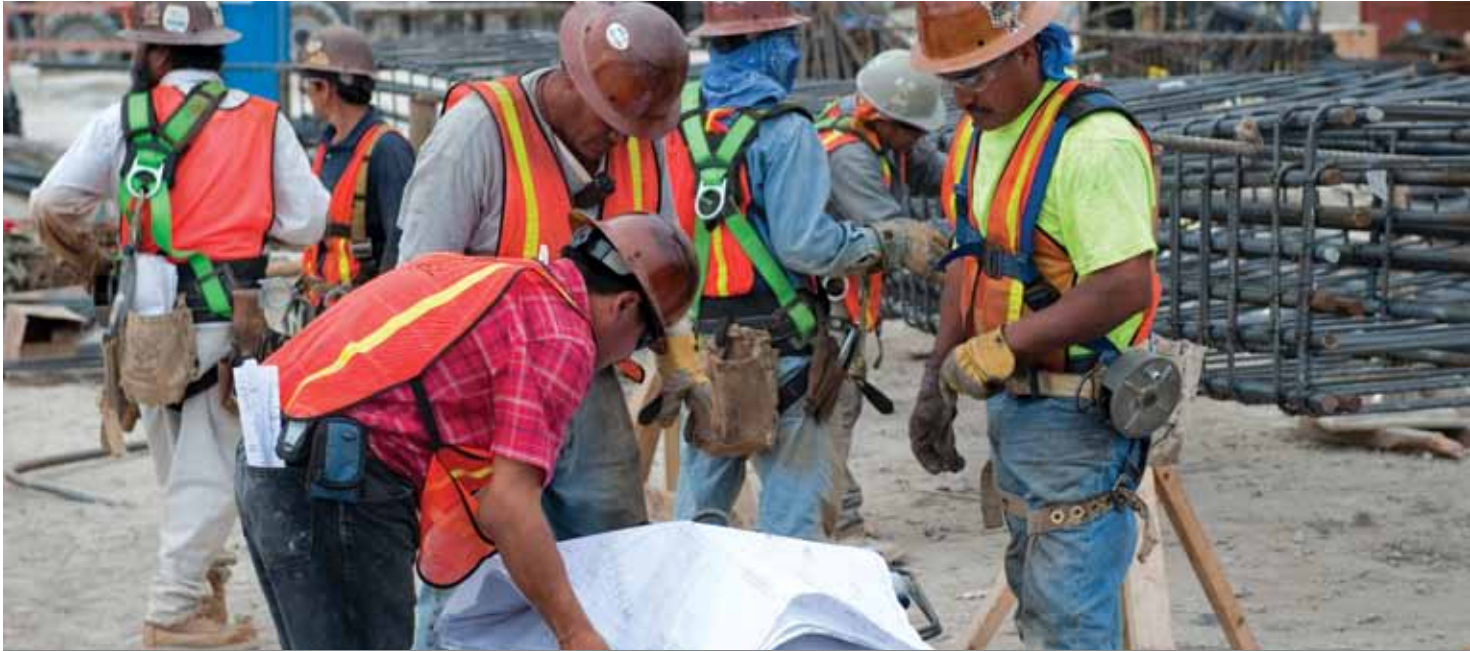
A new Florida Marlins Baseball Ballpark is under construction with a sustainability approach. The ballpark will be accessible via public transportation, will have solar panels on its parking garages, will have accessible seating, and will be applying for Leadership in Energy and Environmental Design (LEED) Silver certification. Five thousand construction jobs are projected by the end of the project and once the Ballpark is open, 2,550 full and part-time jobs are anticipated.
